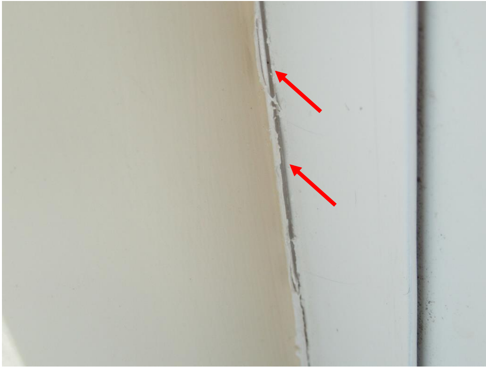
Gapping at the window frame and drywall in unit 101.
