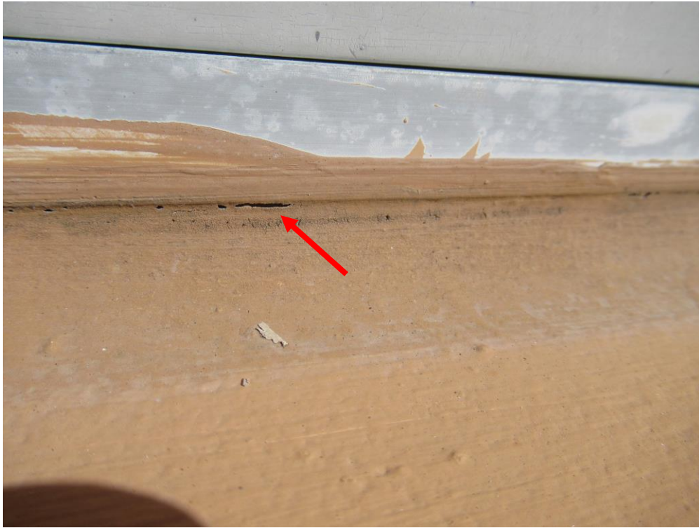
Failing window sealant, unit 101.
