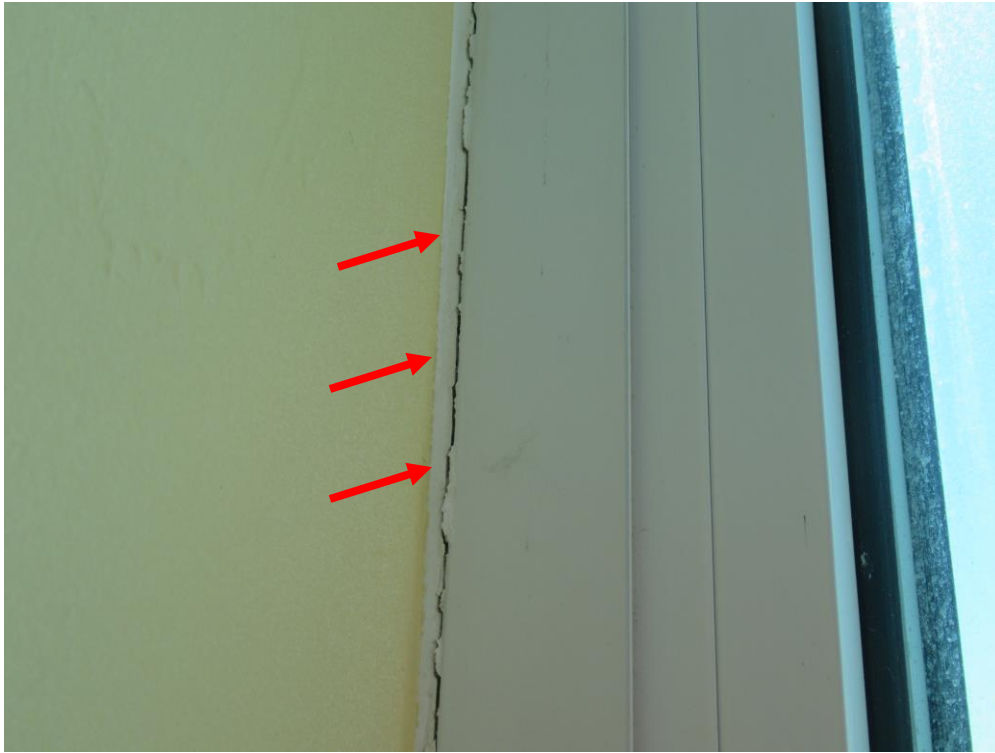
Gapping at the window frame and drywall in unit 303.
