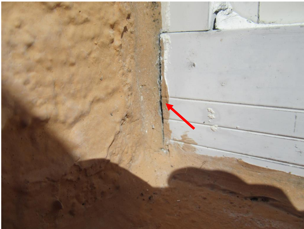
Failing window sealant, unit 102.
