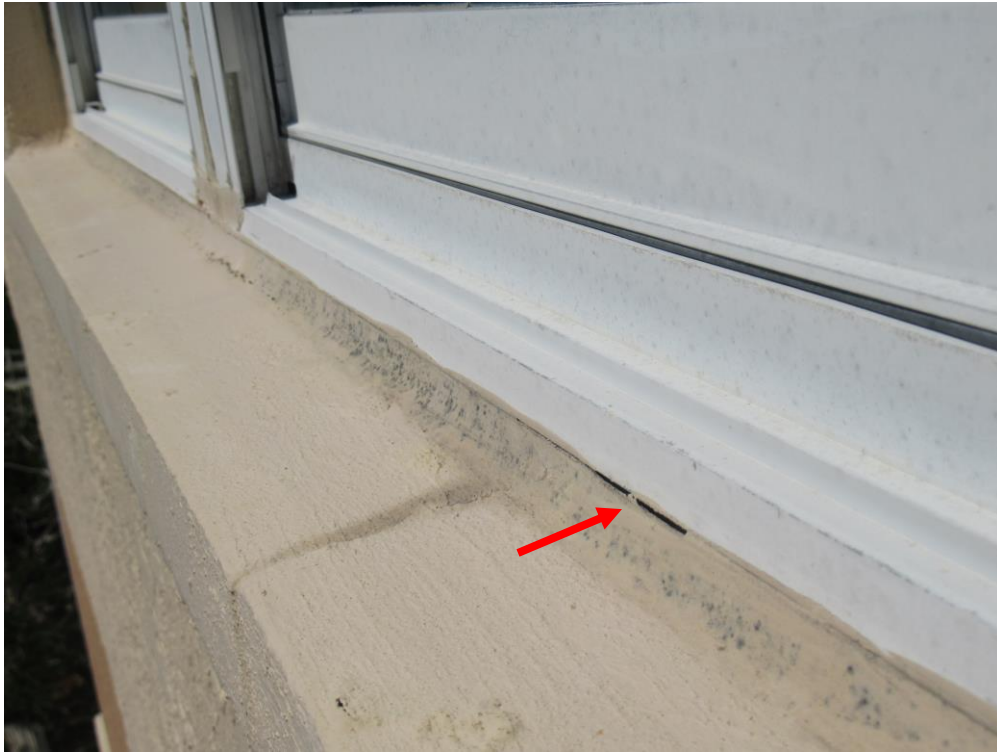
Failing window sealant, unit 307.
