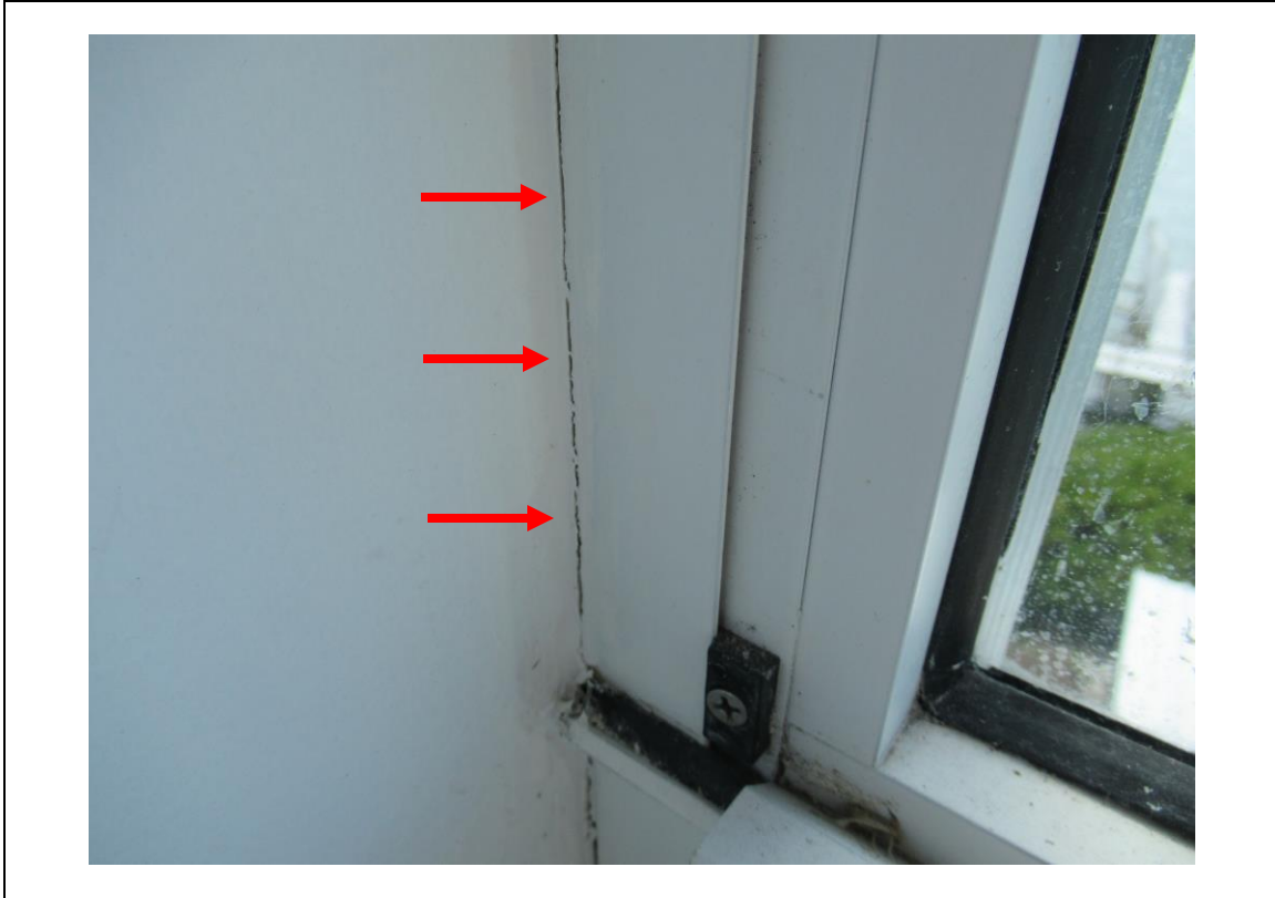
Gapping at the window frame and drywall in unit 301.
