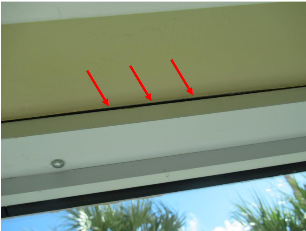
Gapping at window header, unit 101.
