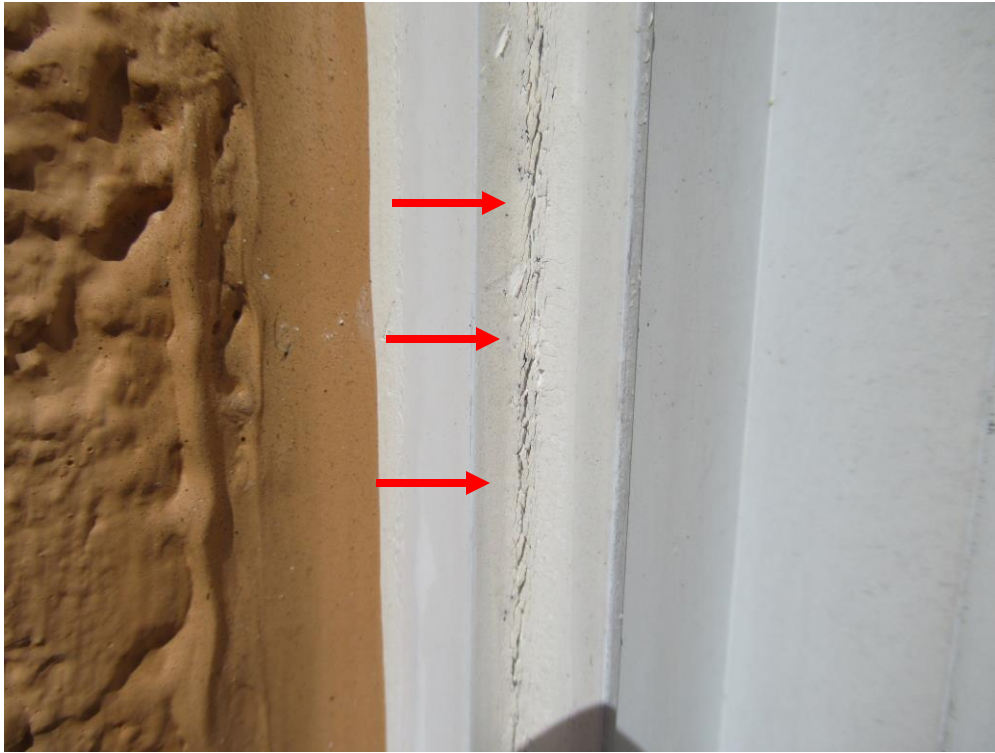
Failing window sealant, unit 106.
