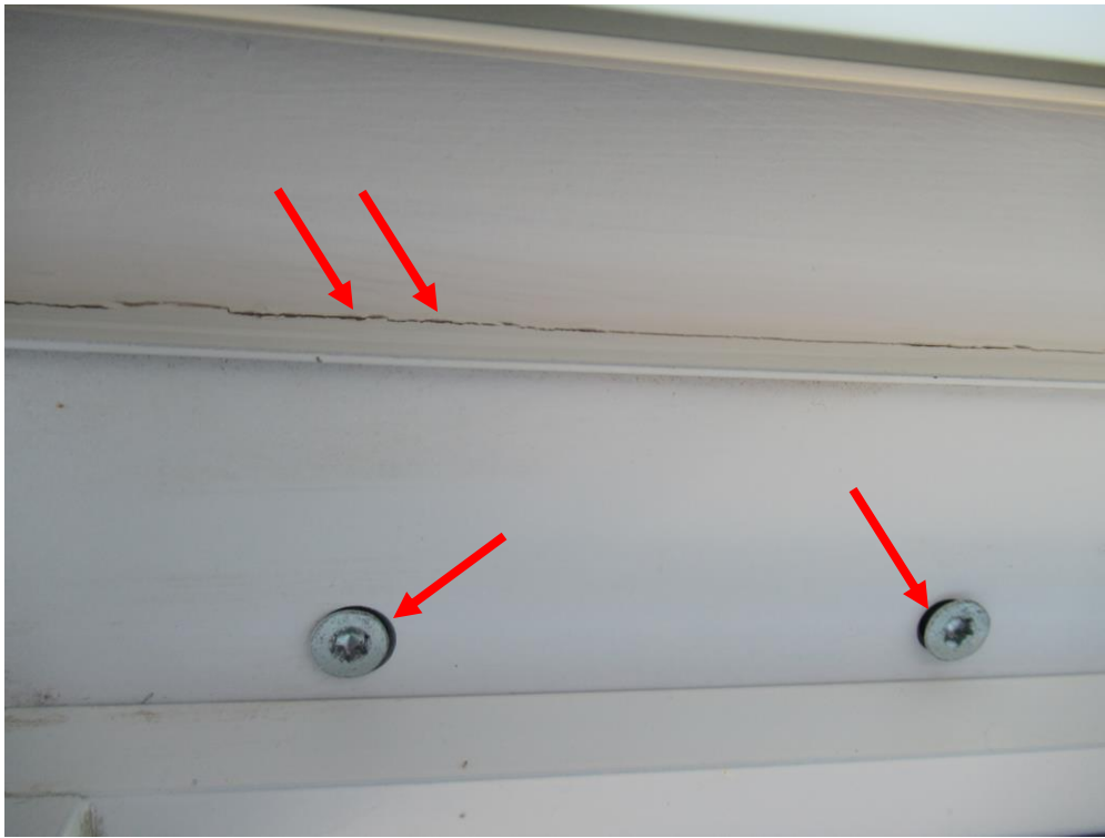
Movement of screws and gapping at the head jamb in unit 107.
