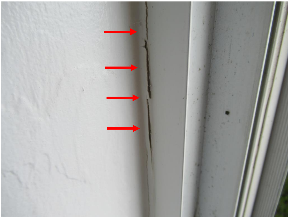
Gapping at the window frame and drywall in unit 301.
