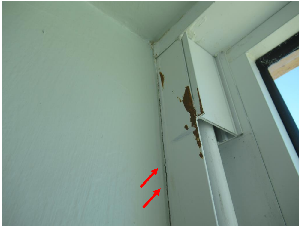
Gapping at the window frame and drywall in unit 107.
