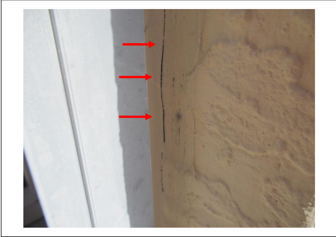
Failing window sealant, unit 301.
