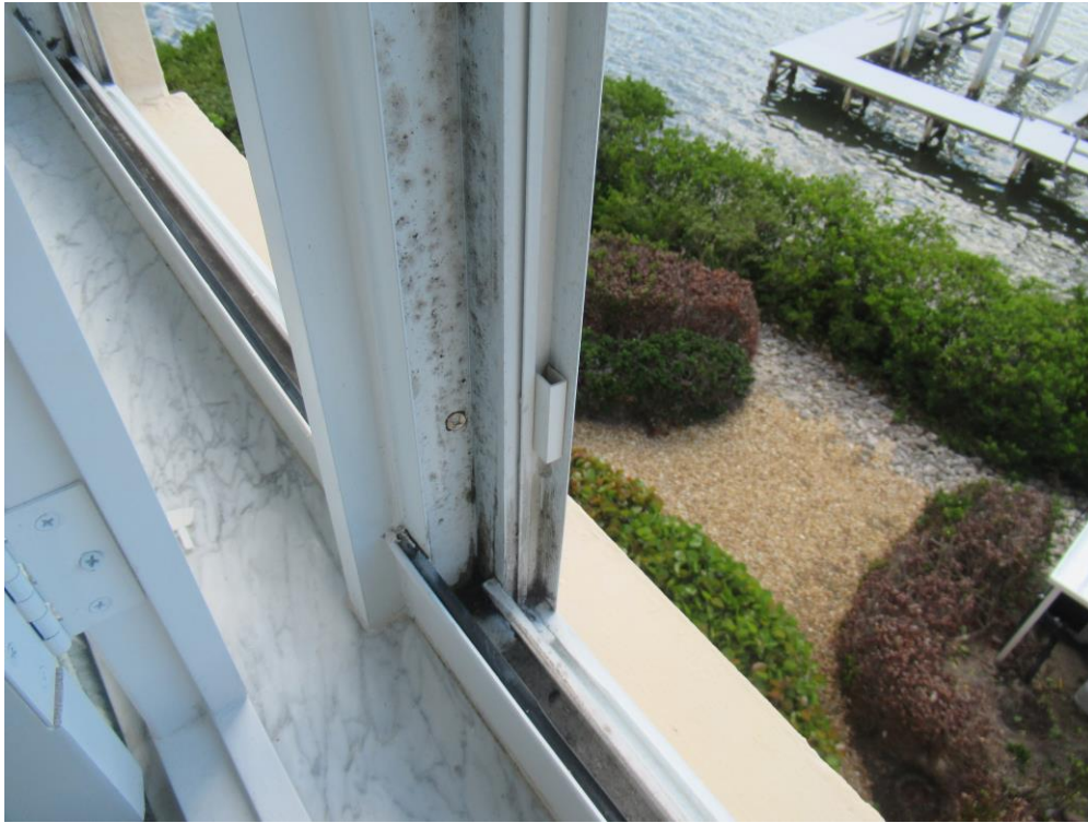
Mold spores in a window track, unit 301.
