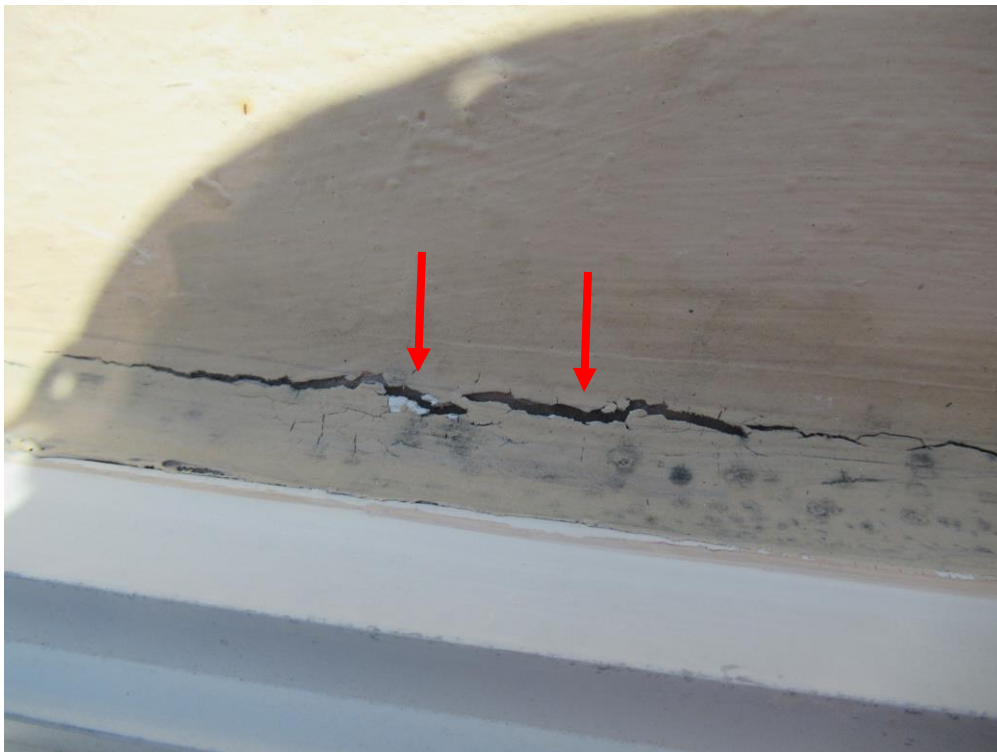
Failing window sealant, unit 506.
