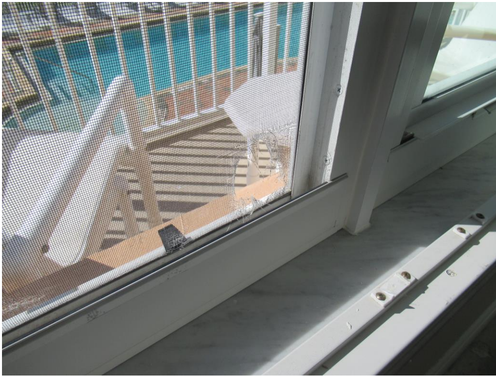
Ripped screen in unit 103.
