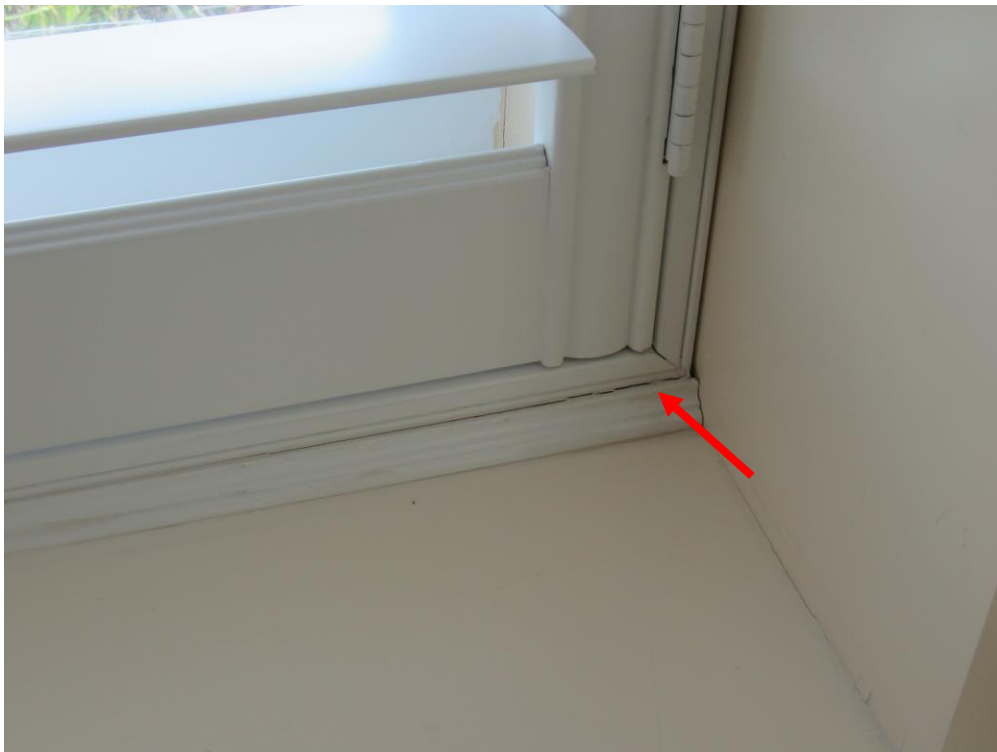
Water damage at plantation shutters, unit 101.
